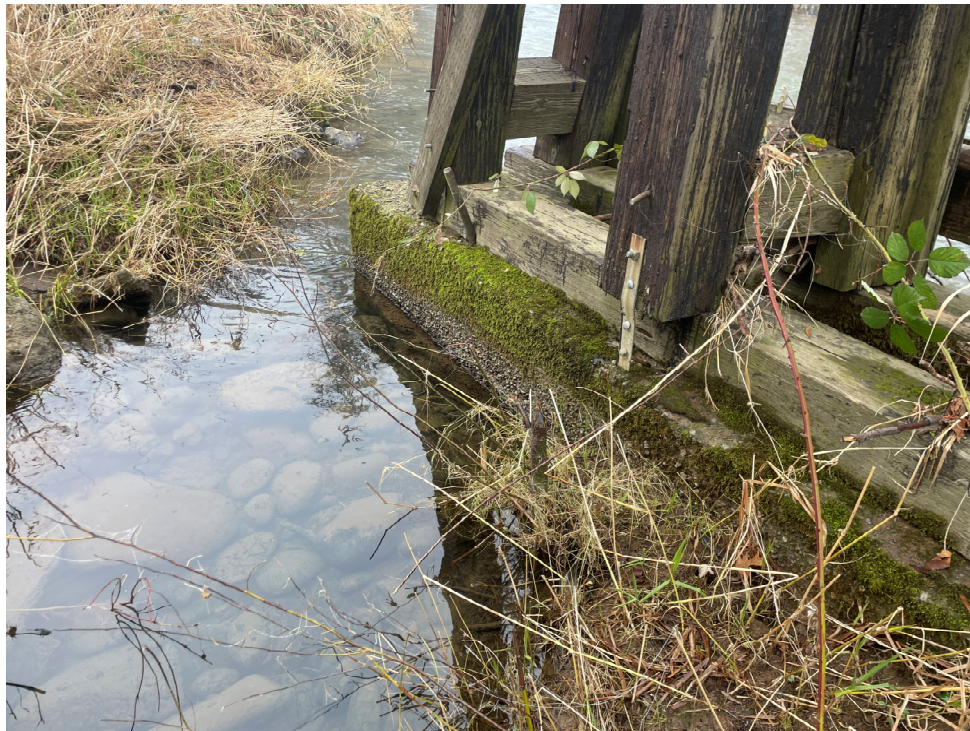
Bent 4B Middle Column Loss of Bearing
