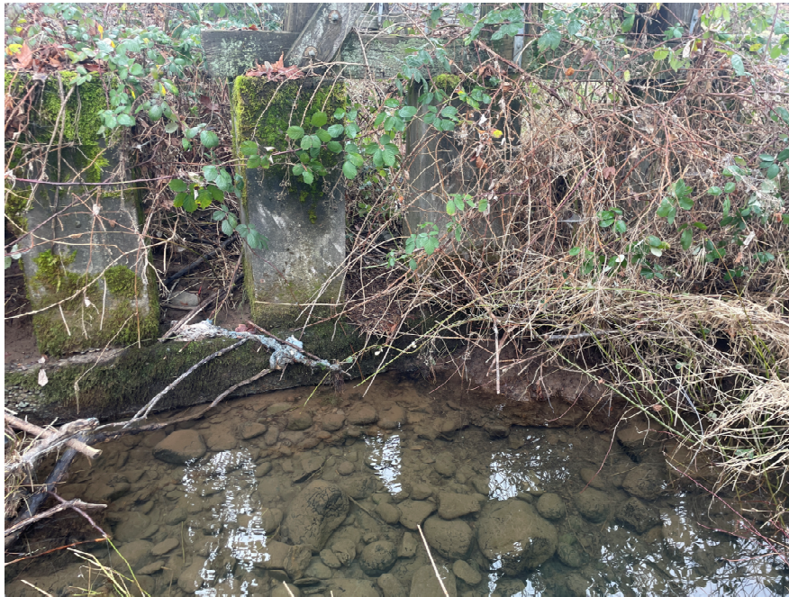
Bent 5 Footing Undermining
