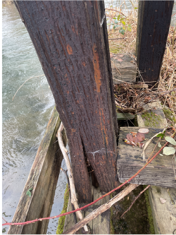
Bent 4A Middle Column Broken
