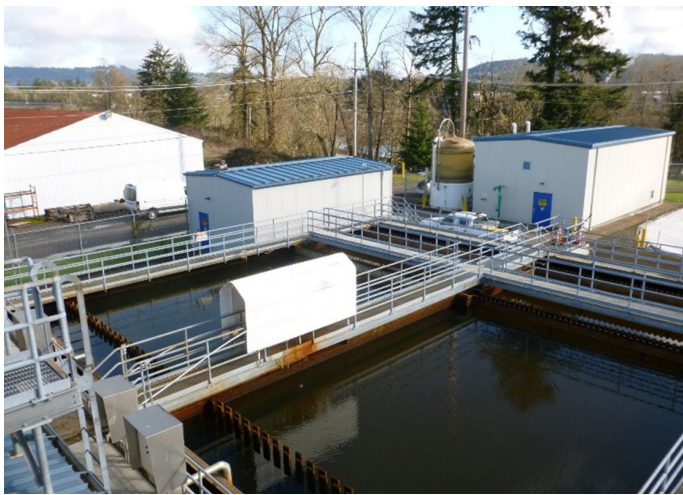
Figure 2: Newberg’s current Water Treatment Plant C. 1953 dilapidated and not in compliance with OHA standards
