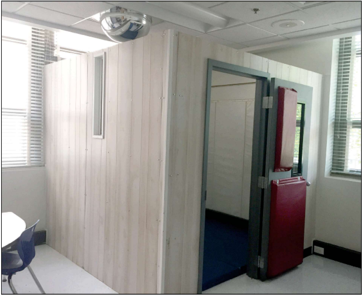
Source: GAO photos. | GAO-20-345
