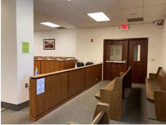
Figure 9: Courtroom #3 - Note beam with green post obstructing the view of spectators/defendants seated in the spectator benches.
