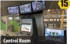
Control Room Total Intelligence Platform combines system controls with data acquisition for real-time insight & optimization
