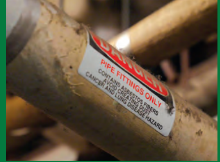
Eradicate asbestos from building for the safety of students, faculty, and staff.
