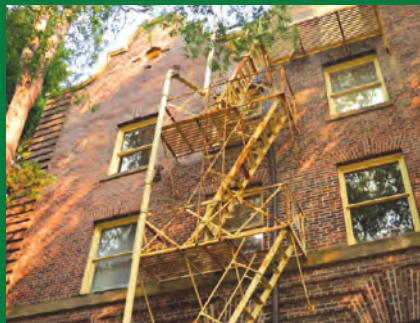
Replace dangerously out-of-date fire egress.
