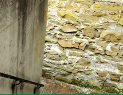
Seismically reinforce this historic building that is rated unsafe for Cascadia earthquake.
