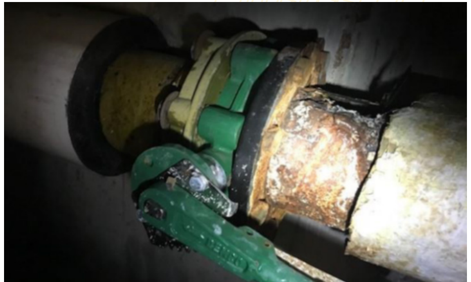
June 2022: Ruptured main line causing temporary campus closure.
