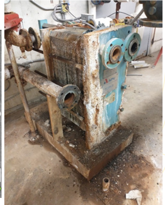
Sept. 2022: Corroded and failed building heat exchanger unit causing temporary building closure.
