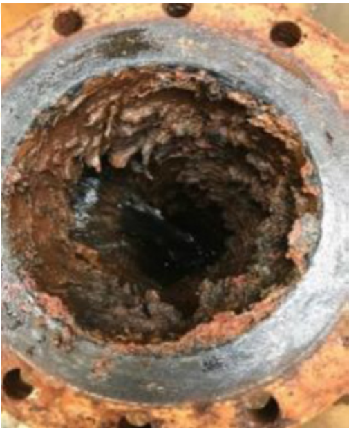
Spring 2022: Corroded and compromised Well #1.
