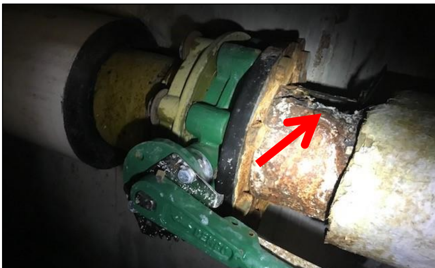
FIGURE 4: RUPTURED PIPE IN TUNNEL
