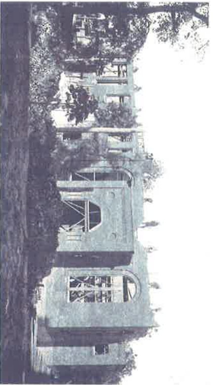
BUILDING A NEW DORMITORY Students draw plans, dig foundations, make the brick, cut timber, which they saw and make into joists and frames. The painting, plastering, plumbing and roofing are also done by the students under the direction of their instructors.
