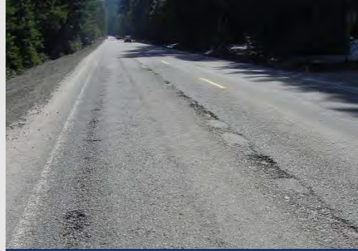
Poor Pavement Conditions
