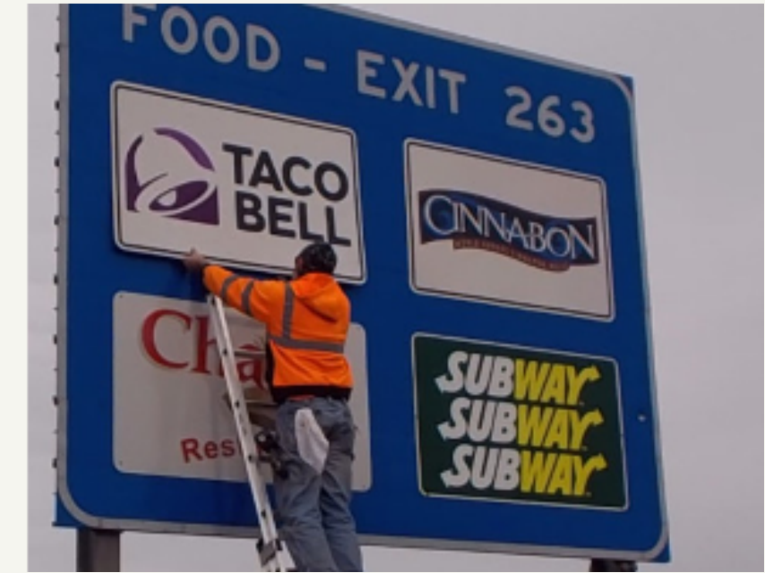
TIC works with 2500 customers, managing 5000 signs
