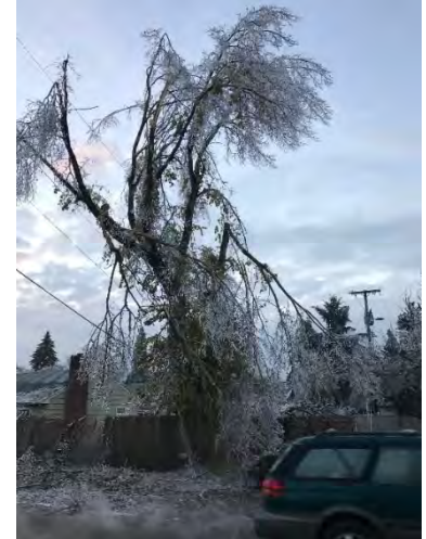
Winter storms can result in area wide outages due to damage to electrical equipment.
