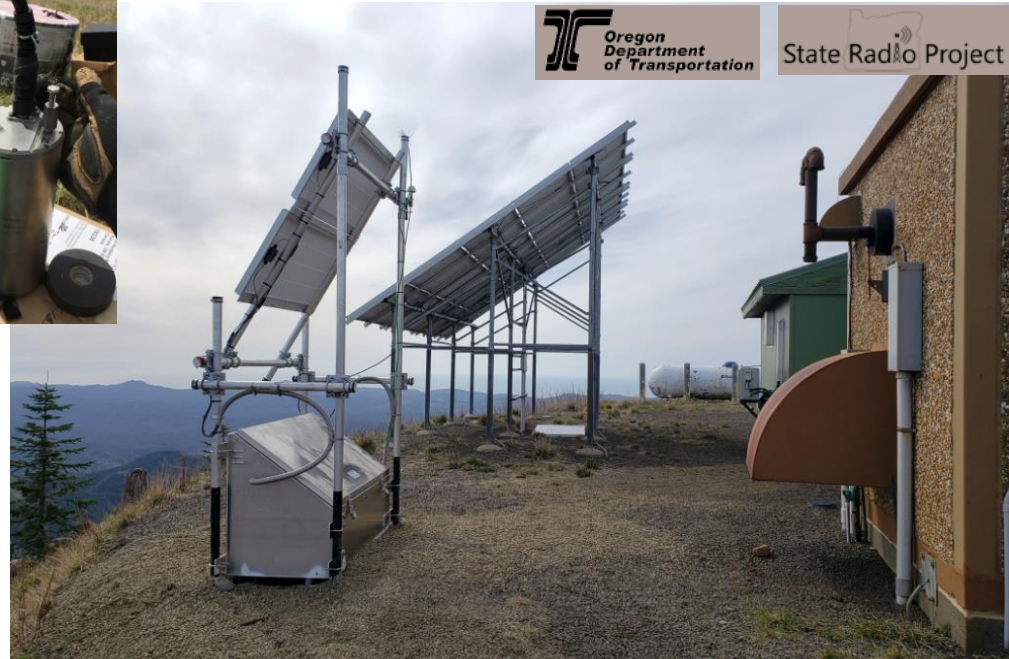
Euchre Mountain seis station: collocated at ODOT-SRP site, state microwave backhaul
