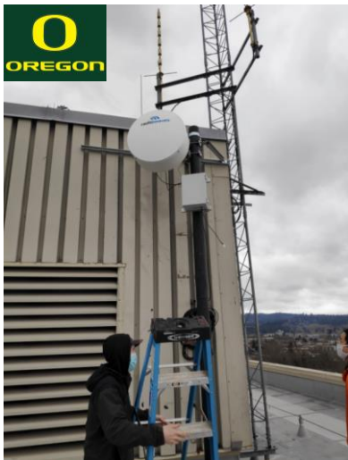
UO rooftop microwave: Receive hub for 6 seis stations
