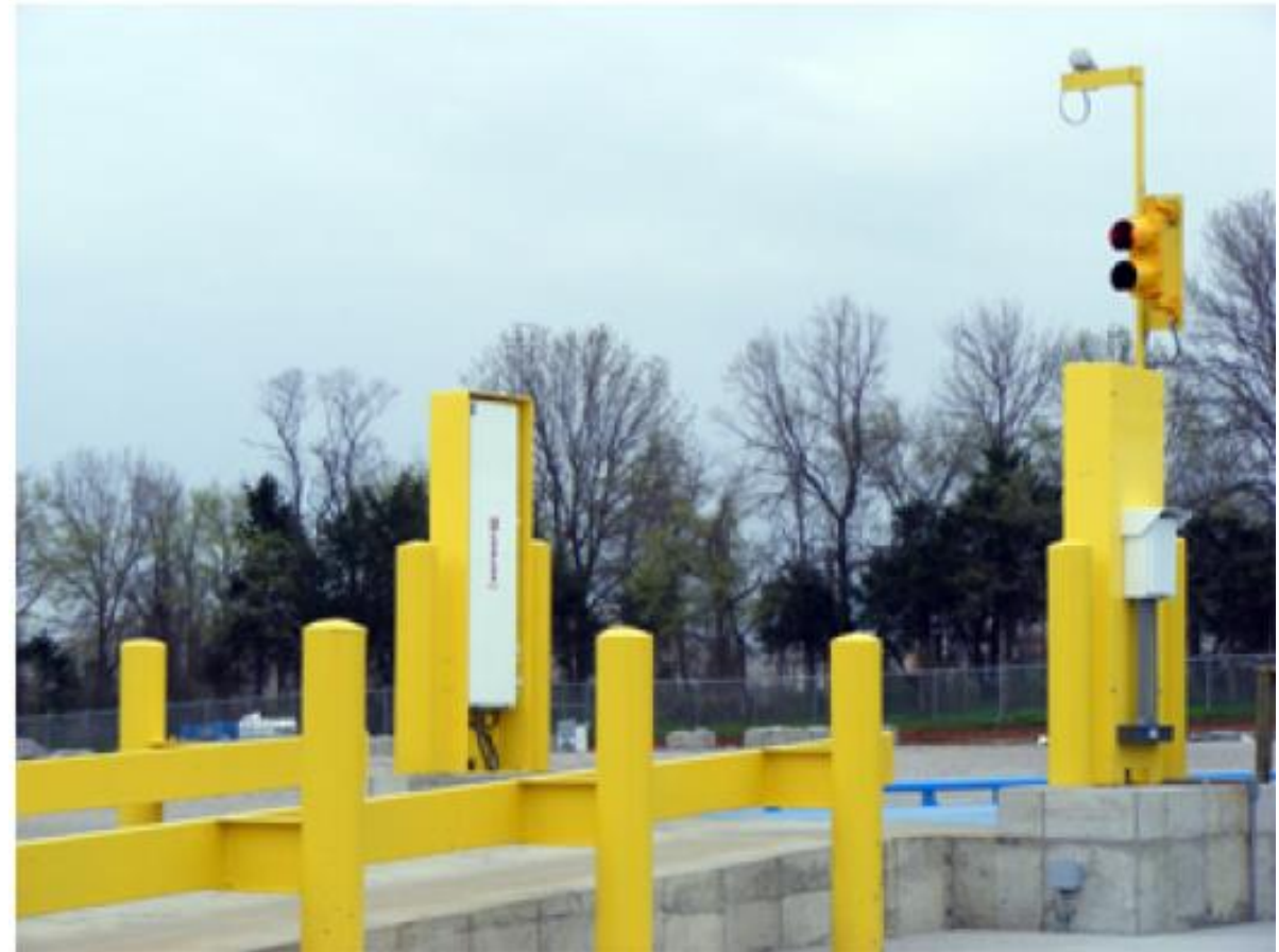
Drive-Thru Radiation Detecting Portal Monitor
