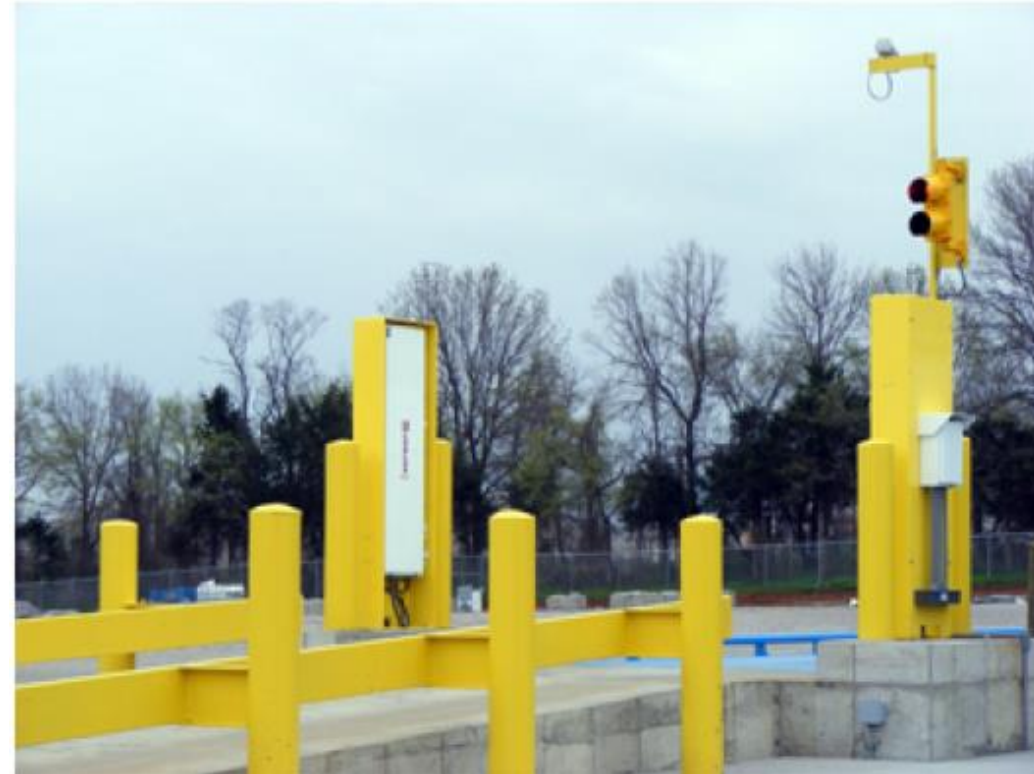
Drive-Thru Radiation Detecting Portal Monitor
