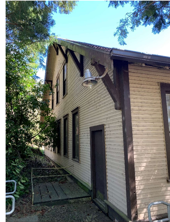
Clackamas Complex Building 4 Currently used by N Willamette District and Fish Research. Was the Hatch House for the former fish hatchery.
