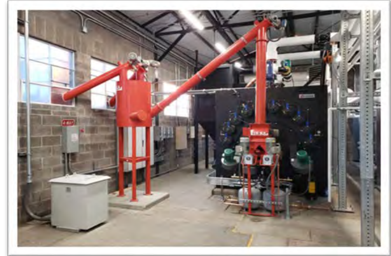
Woody biomass pellet boiler
