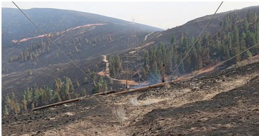
Wildfire knocked out BPA's Hot Springs-Rattlesnake 230-kV line in Montana in August 2015 46
