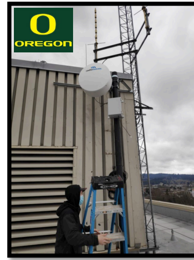
UO rooftop microwave receive hub
