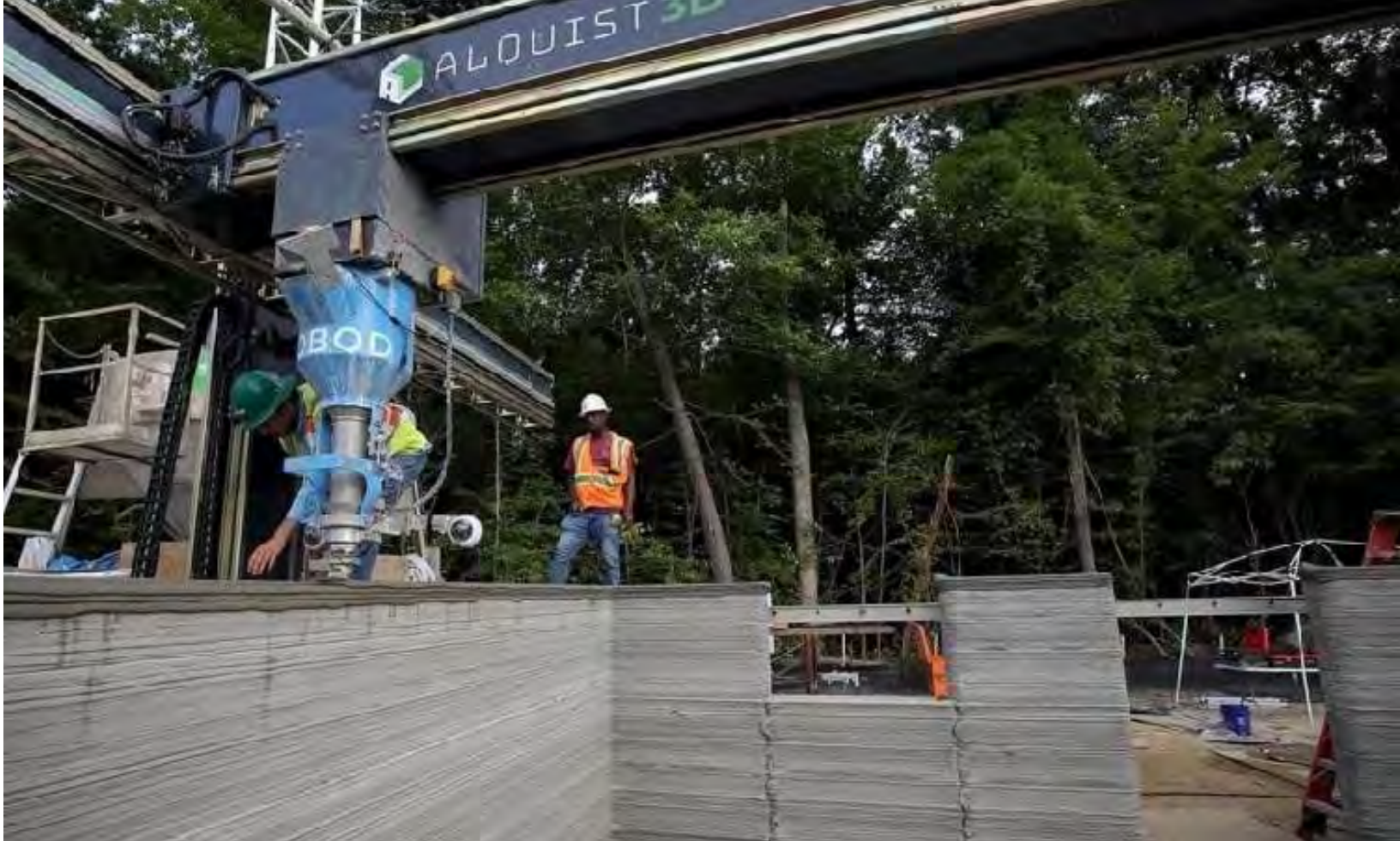
The first 3D printed homes in Oregon will be The Ridge in John Day, a master-planned development overlooking the John Day River. The Ridge will provide veteran's preference housing at a target rental rate of $850 per month. Photo: John Day Facebook page
