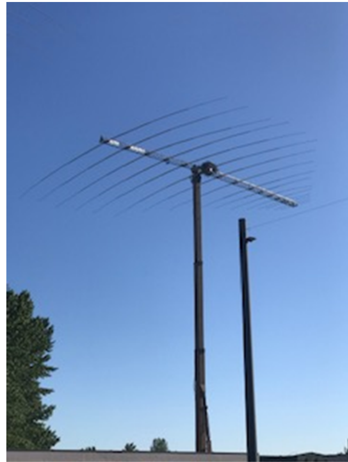
Joint Operations Center HF Antennas
