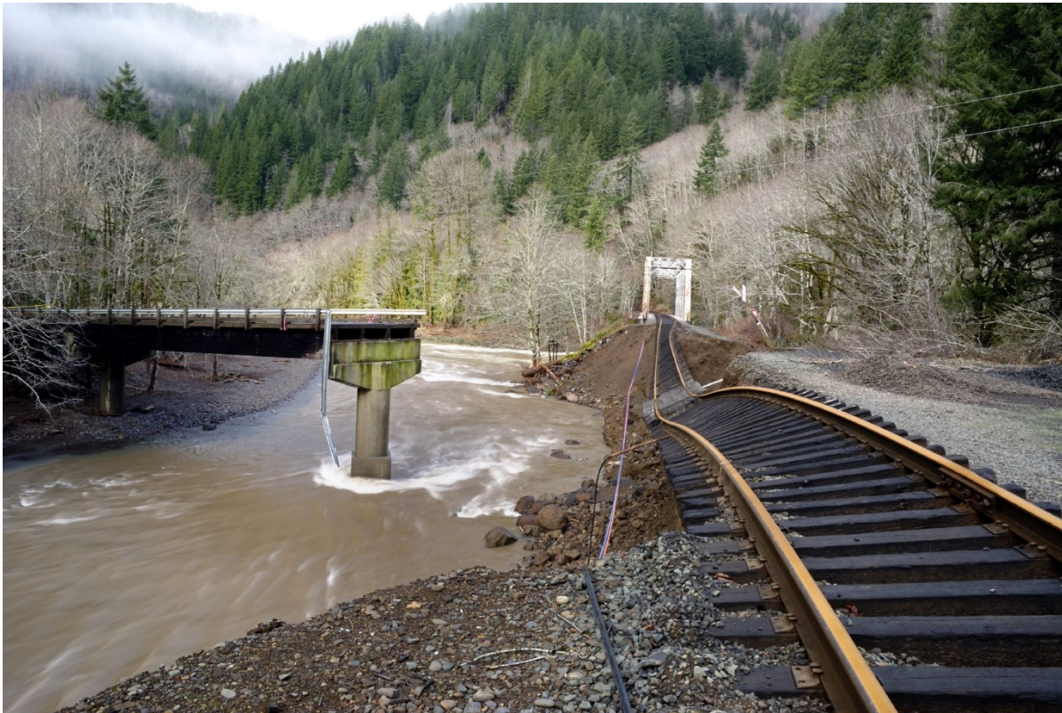
Figure 2: Damage to the Port of Tillamook Bay railroad from channel migration of the Salmonberry River (Courtesy Chris Updegrave, 2/9/2008, https://www.flickr.com/photos/cupdegrave/2253462031/in/photostream/ )
