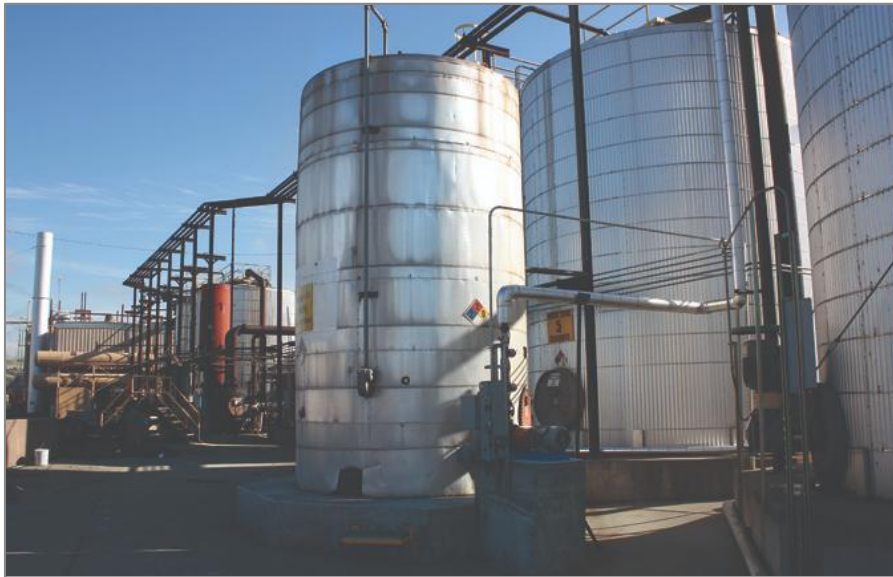
Creosote storage tanks at the AmeriTies plant. (Jesse Burkhardt/The Dalles Chronicle)
