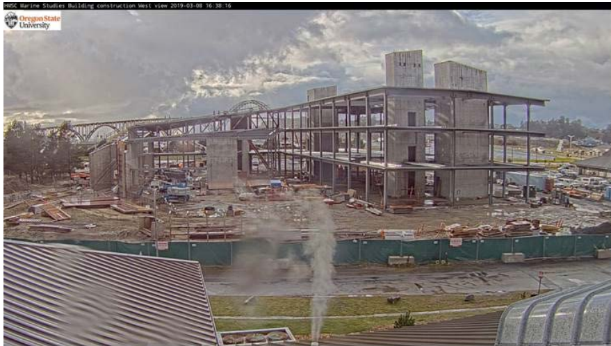
Tsunami vertical evacuation building that is currently under construction by OSU in Newport. Source: http://webcam.oregonstate.edu/msisouth 3/8/19
