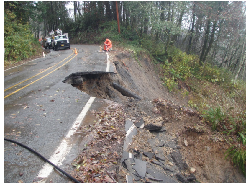
Carpenterville Highway No. 255 A portion of the highway washed out in December 2015
