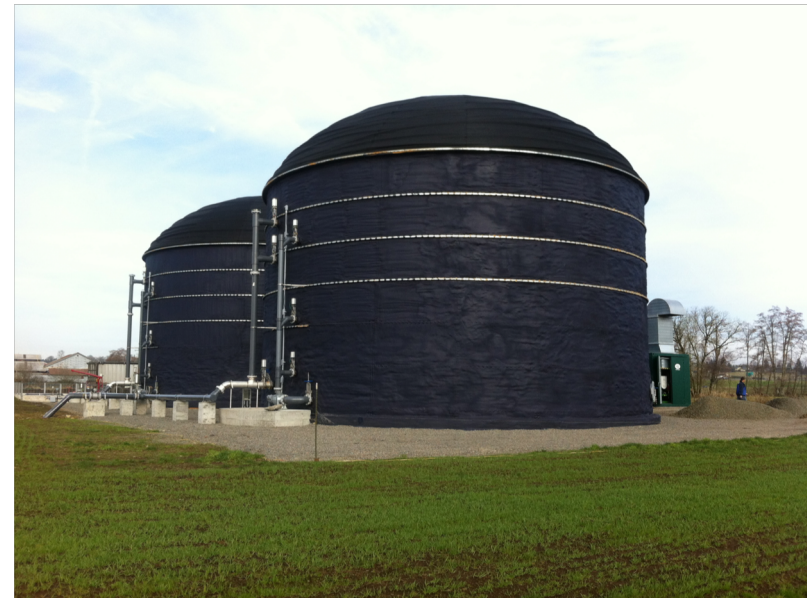
Oak Lea Dairy Digester, Aumsville, Oregon
