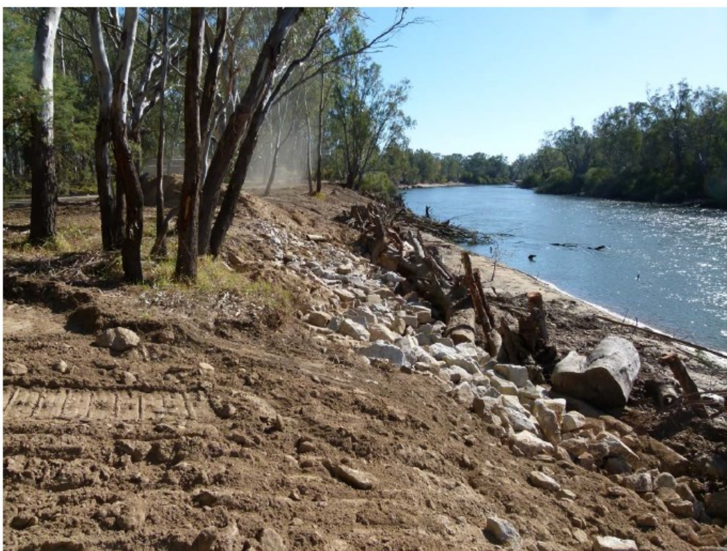
Figure 13: Ball Park log revetment being repaired and retro-fitted with rock beaching and backfilled.
