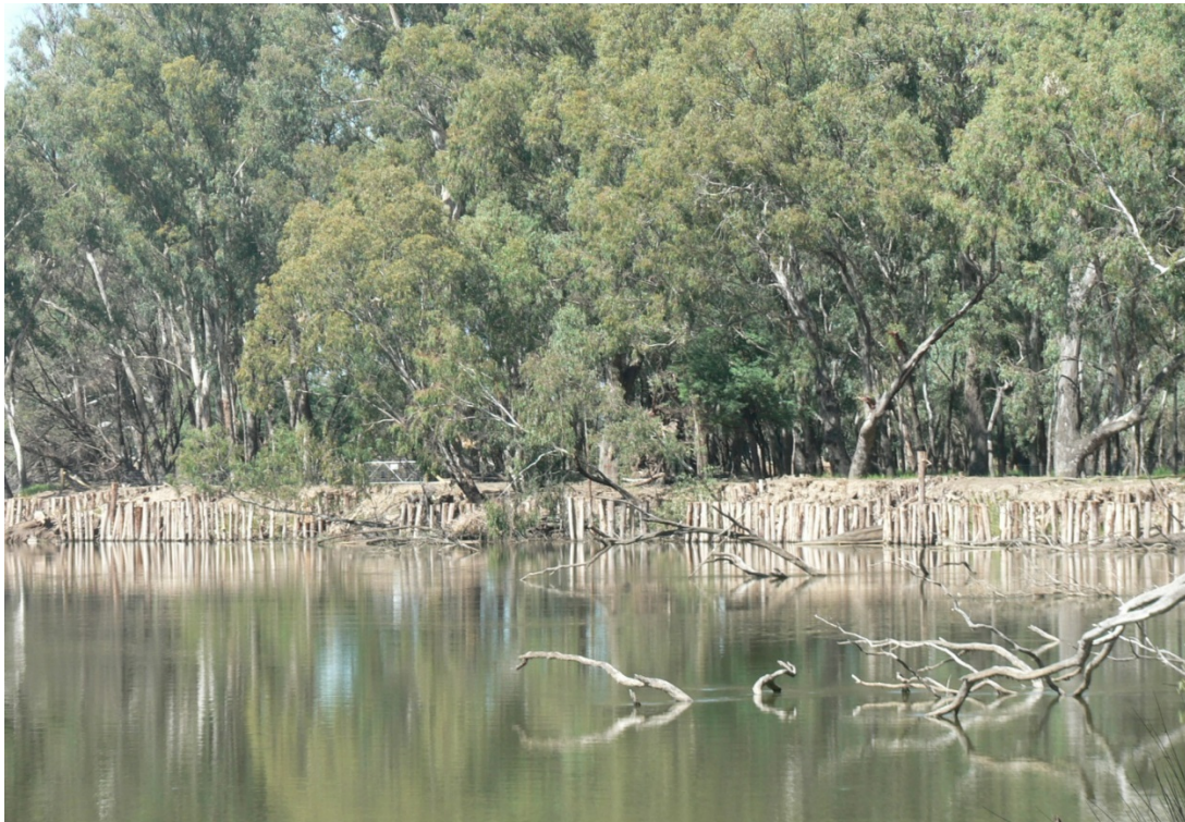
Figure 3: Pile fields are one type of river work technique implemented to reduce rates of erosion. These structures were designed to be sympathetic to the natural behaviour of the river. They are ineffective at addressing erosion caused by boat waves as these wave travel perpendicular to the bank.
