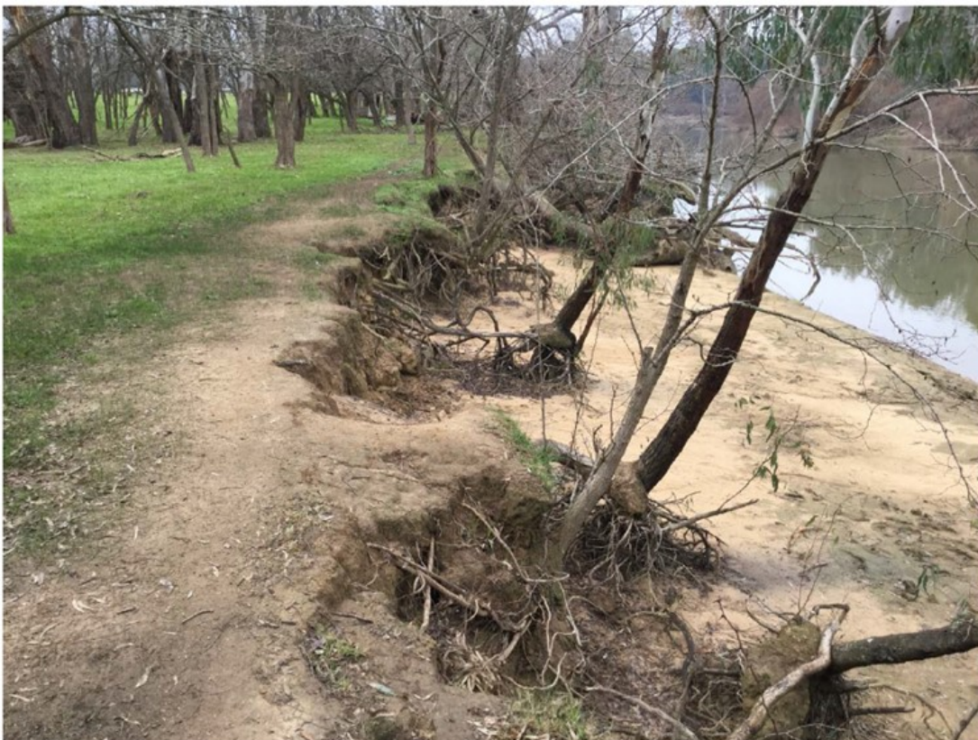
Figure 4: Erosion near Corowa that is typical of the impacts of boating.
