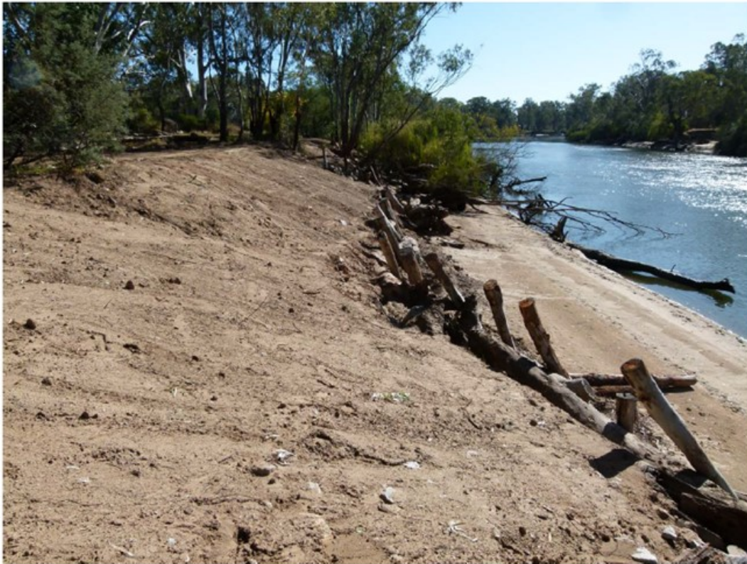
Figure 14: Ball Park logs now repaired with the aim of being able to withstand the impact of vessel wash.
