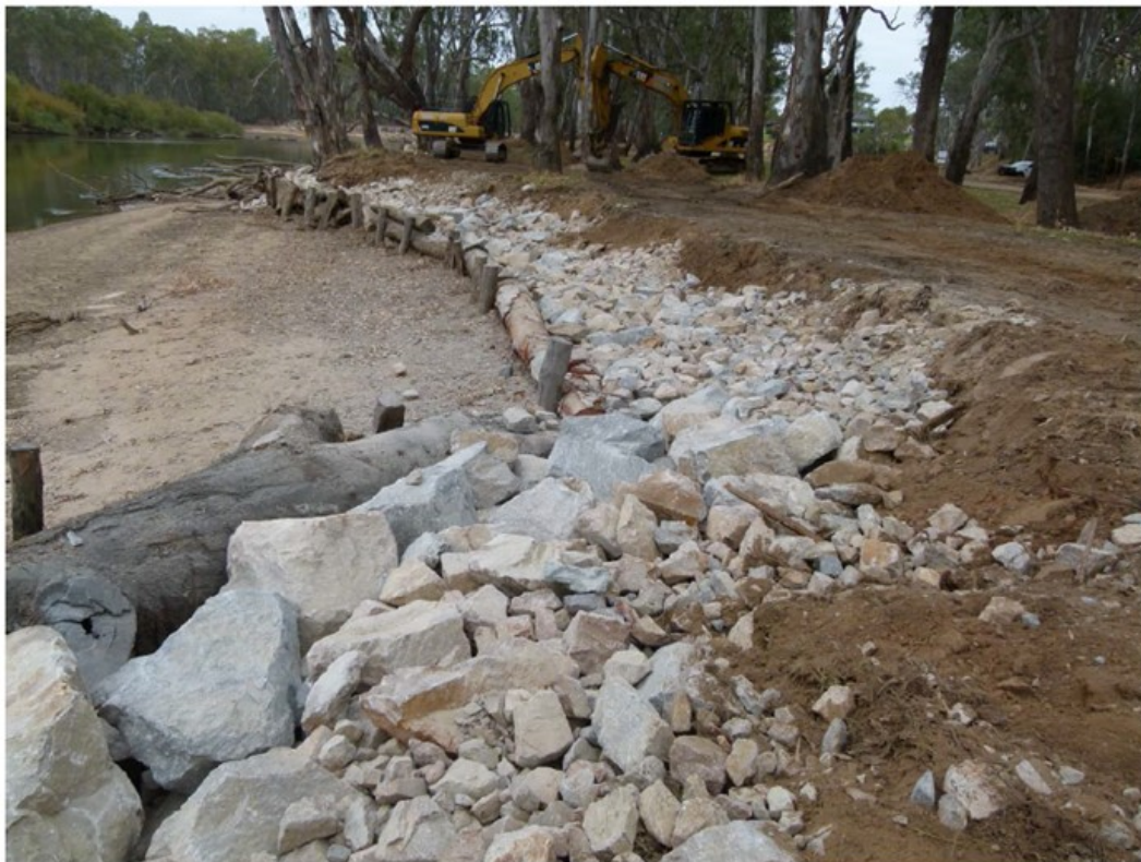
Figure 12: Retrofitted rock beaching behind the log revetment to protect against vessel wash. Note the elongated sloping ledge - a common feature seen in areas that are subjected to high levels of vessel wash, where the upper vertical face retreats much faster than the toe of the bank.
