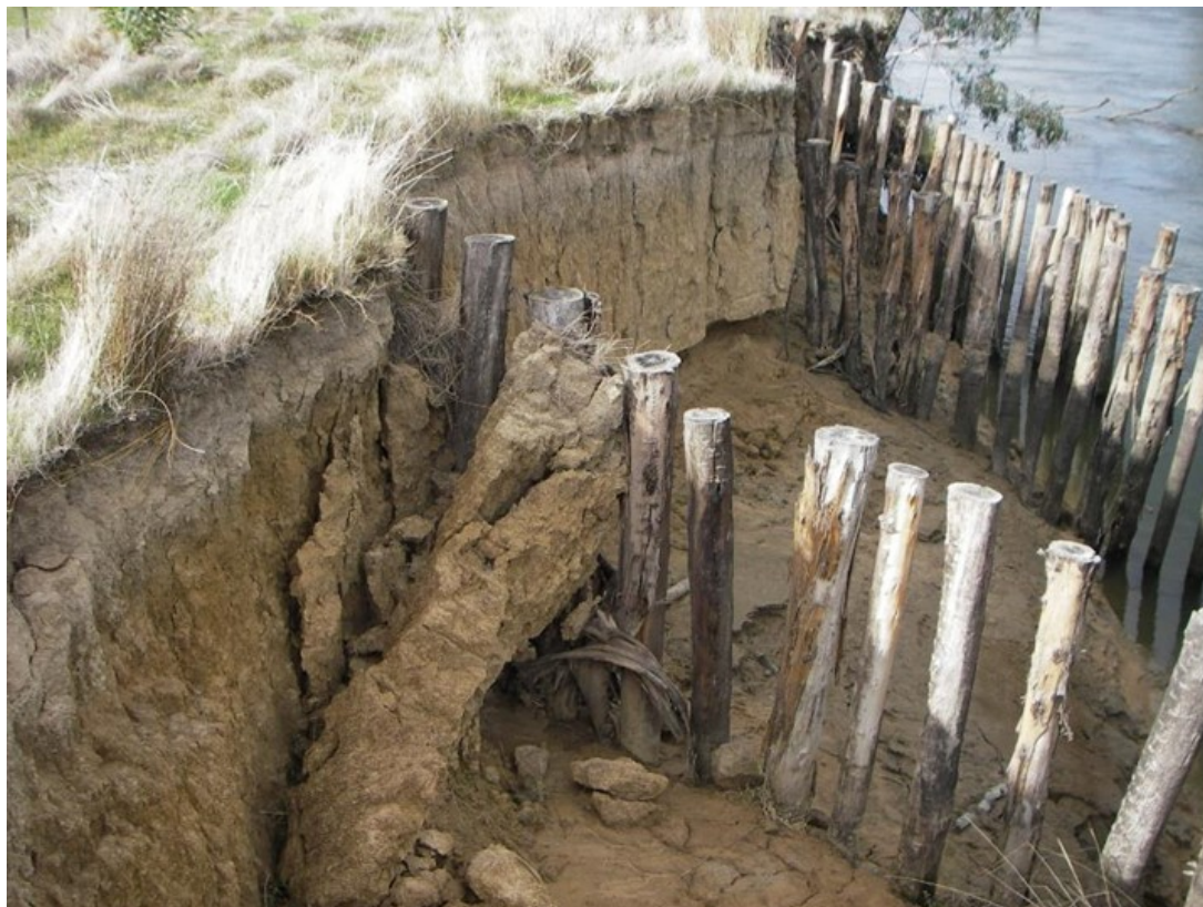
Figure 18: Bank sheering behind pile fields.
