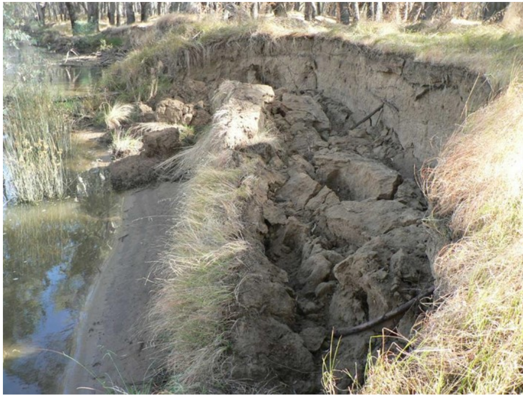
Figure 17: Severe bank slumping of grassy bank face.
