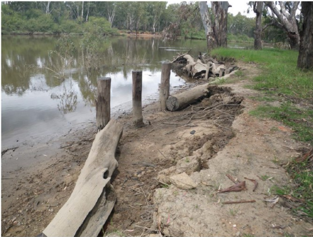
Figure 10: Undermined log revetment leading to ongoing retreat of the upper bank.
