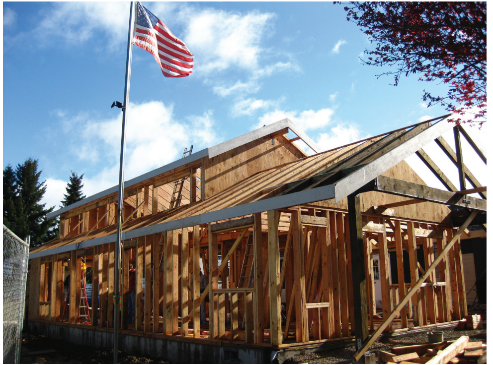
The Village Apartments were extensively remodeled using Housing Preservation Funds provided by Oregon Housing and Community Services.
