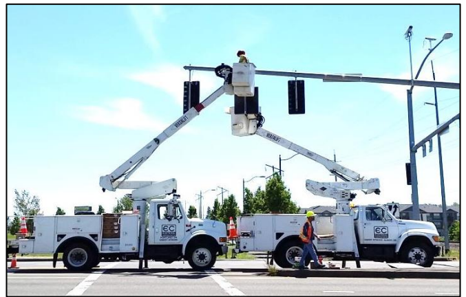
IBEW Electricians operating bucket/boom trucks while working on traffic signal near Keizer Station 5/23/17
