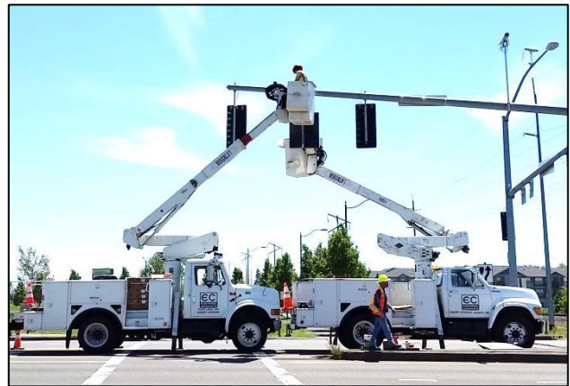
IBEW Electricians using bucket/boom trucks while working on traffic signal near Keizer Station 5/23/17
