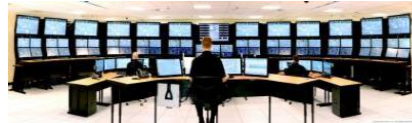
NuScale Control Room Simulator
