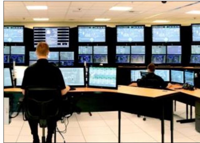
NuScale Control Room Simulator
