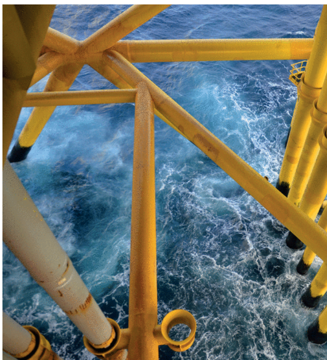
An up-close look at the Valemon platform, one of Statoil’s stand-alone development projects on the Norwegian continental shelf.
