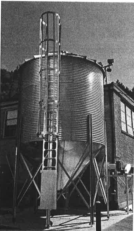
OREGON-MADE A number of the new biomass heating systems, such as this one at Oakridge Elementary School, are manufactured in Oregon by SolaGen Inc., which is based in St. Helens.
