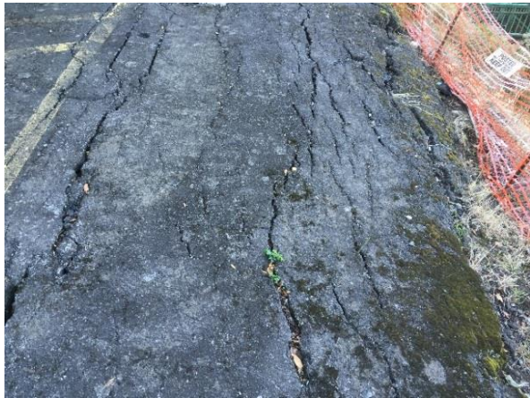
Eroding asphalt at Willamette River elevation
