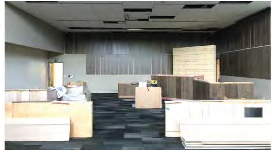
View of a partially constructed courtroom in the new Jefferson County courthouse.
