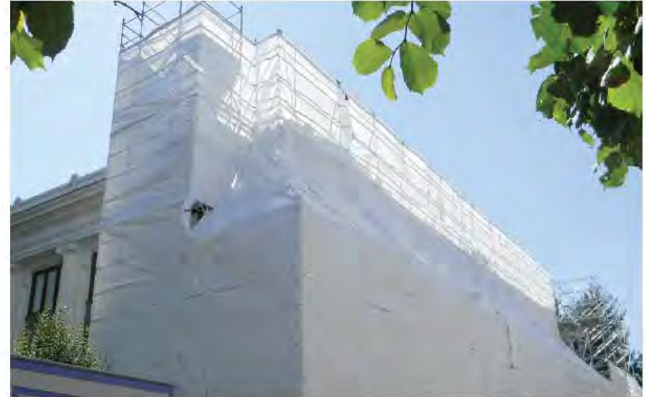
Supreme Court Building scaffolding on the north facade is draped with dust covering during rehabilitation work.
