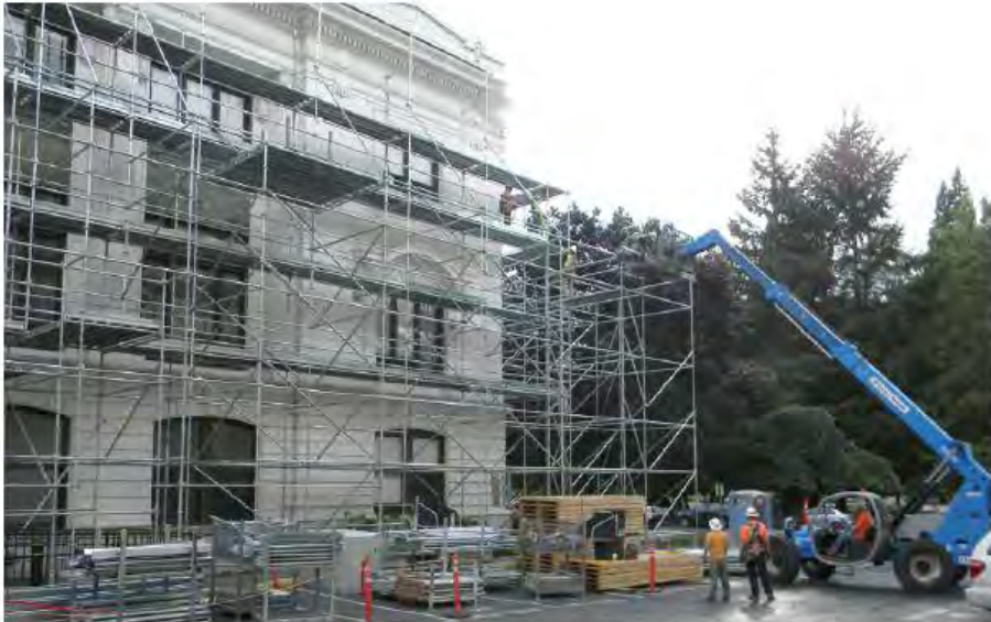
Workmen build scaffolding support system on the north facade of the Supreme Court Building, in preparation for rehabilitation work on the exterior of the building.
