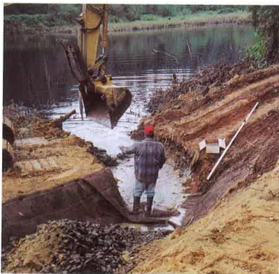
Fish will pass through this new channel to a large pond and several streams that drain into Hall Slough.
