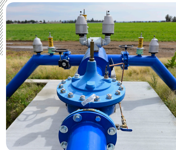
Pressurized water delivery means this irrigation district patron no longer needs to pump water out of a canal. In fact, the excess pressure at this site may be able to support a small hydro turbine in the future.
