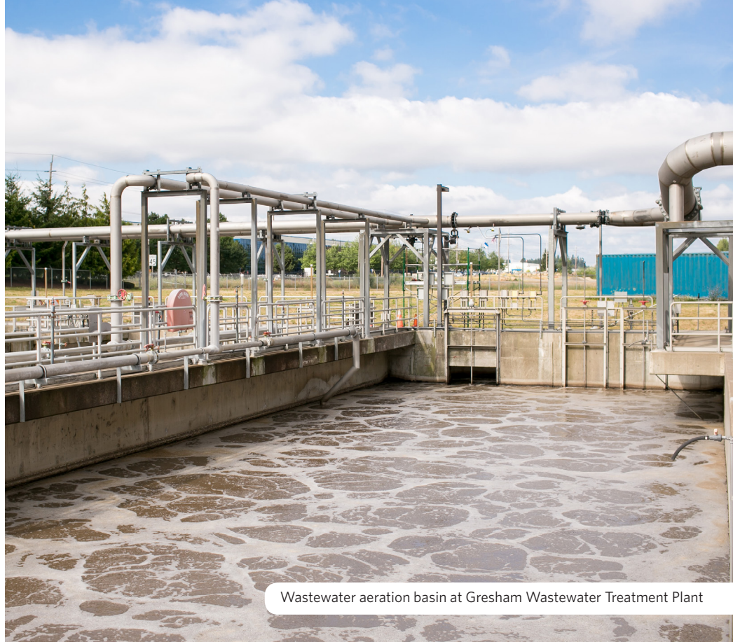
Delivering FOG to Gresham Wastewater Treatment Plant
