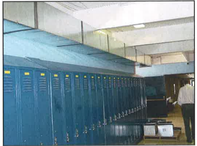
Klamath County School District installed new ducts at Henley High School and added insulation to the exterior walls and ceiling to reduce heat loss to the building constructed in 1968.
