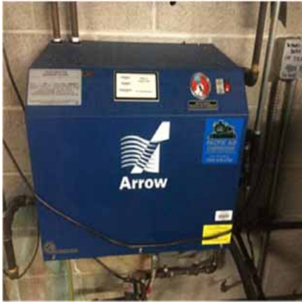
D2099 Other Piping Systems.3:- View of the air dryer unit.
