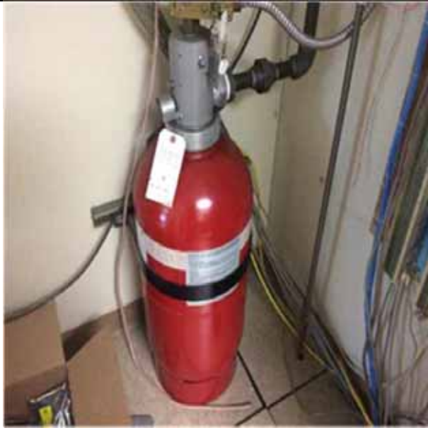
D4091 Carbon Dioxide Systems.1:- View of the clean agent storage tank.
