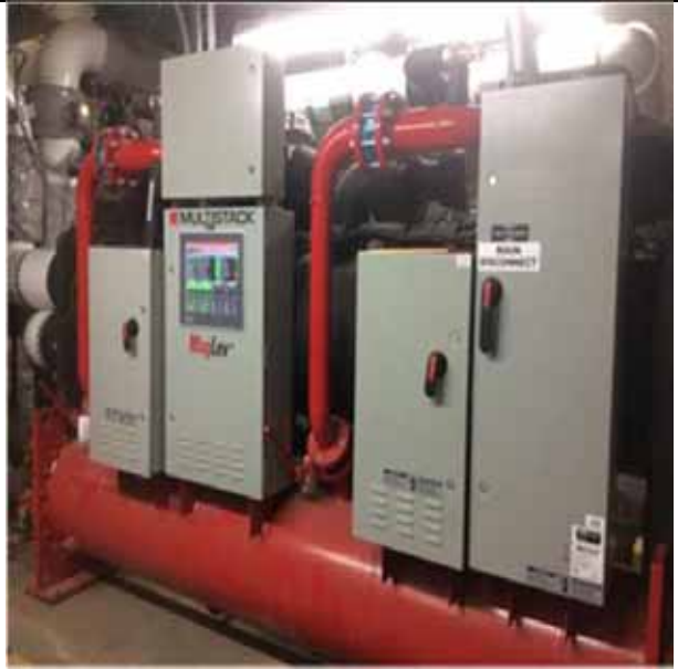
D3031 Chilled Water Systems.1:- View of chiller CH-01.
