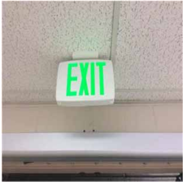
D5092 Emergency Light & Power Systems.2:- View of a typical emergency exit light sign.
