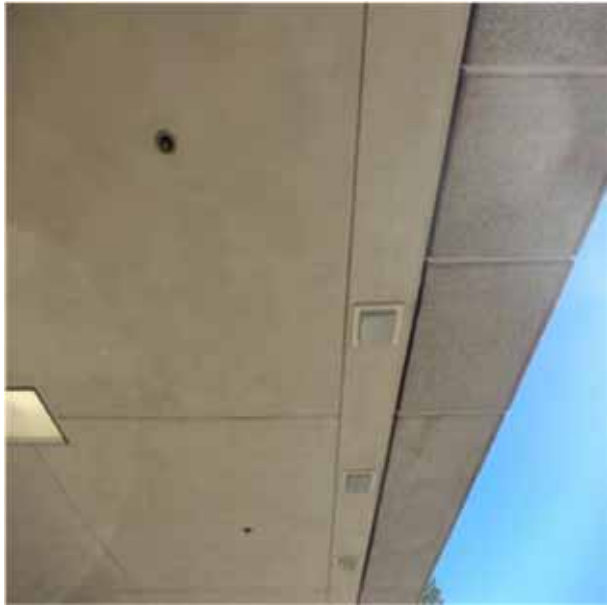
D5022 Lighting Equipment.3:- View of the smaller 1' x 1' light fixtures at the exterior soffits.
