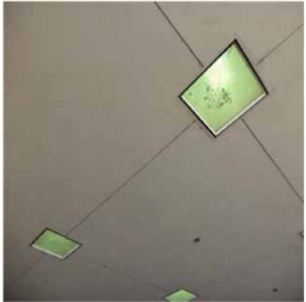
D5022 Lighting Equipment.4:- View of the 2' x 2' light fixtures at the exterior soffits.
