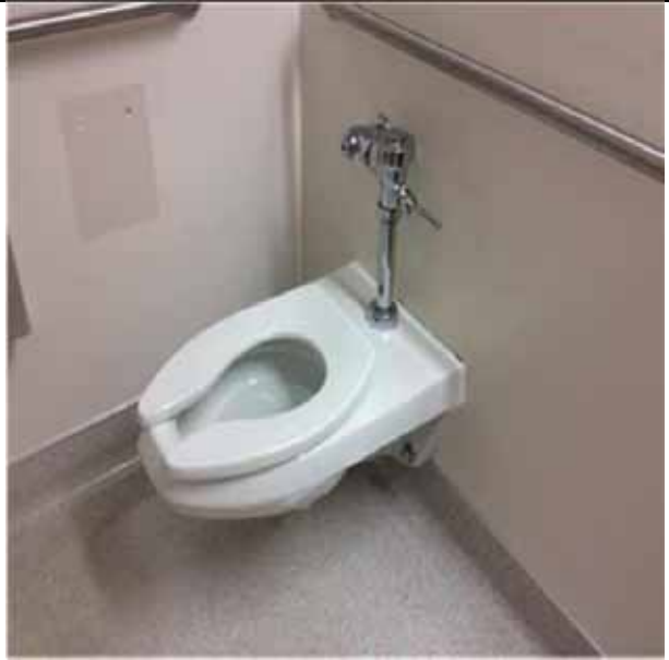
D2011 Water Closets.1:- View of the wall mounted water closets.
