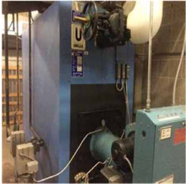
D3021 Boilers.1:- View of the HVAC boiler.
