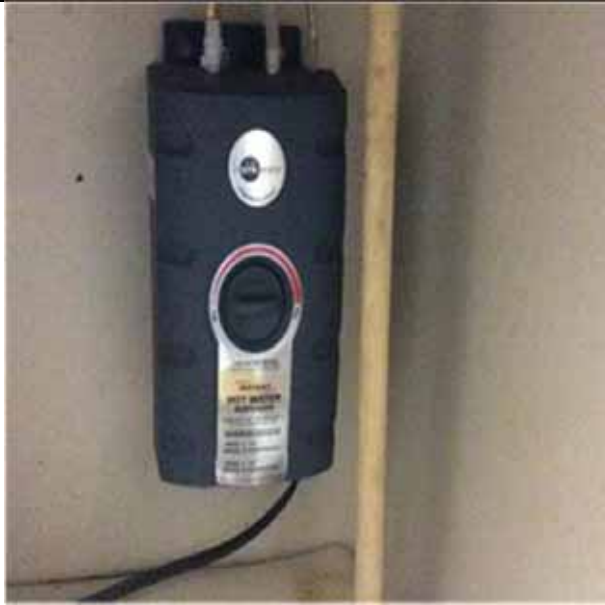
D2022 Hot Water Service.3:- View of one of the point-of-use water heaters.
