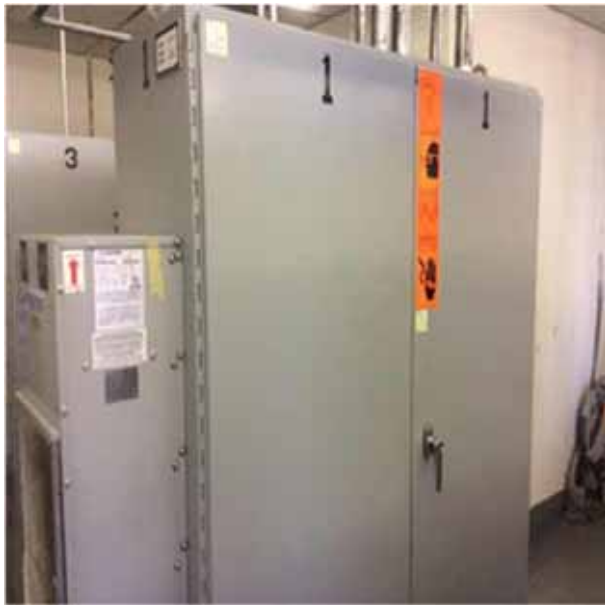
D1011 Passenger Elevators.2:- View of the controller unit for elevator 01P.
