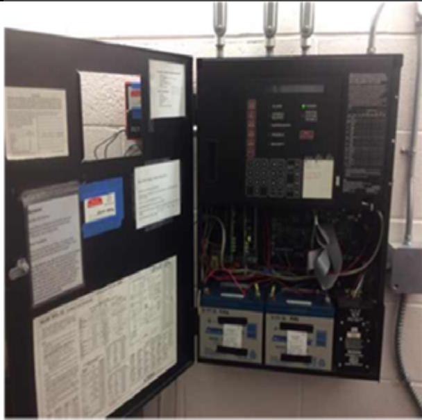
D5037 Fire Alarm Systems.1:- View of main FACP.
