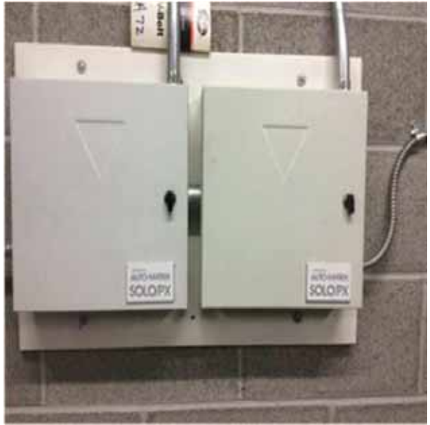
D3068 Building Automation Systems.1:- View of the BAS control unit.
