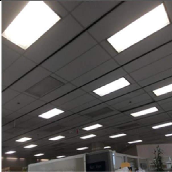
C3032 Suspended Ceilings.1:- View of typical acoustic ceiling system.
