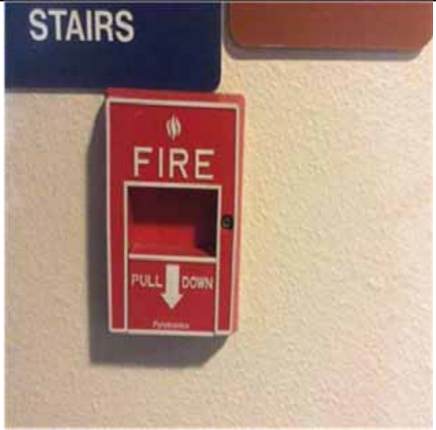
D5037 Fire Alarm Systems.2:- View of a fire alarm pull box device.
