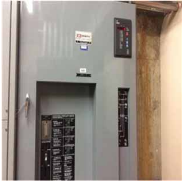
D5012 Low Tension Service & Dist.5:- View of one of the emergency transfer switches.
