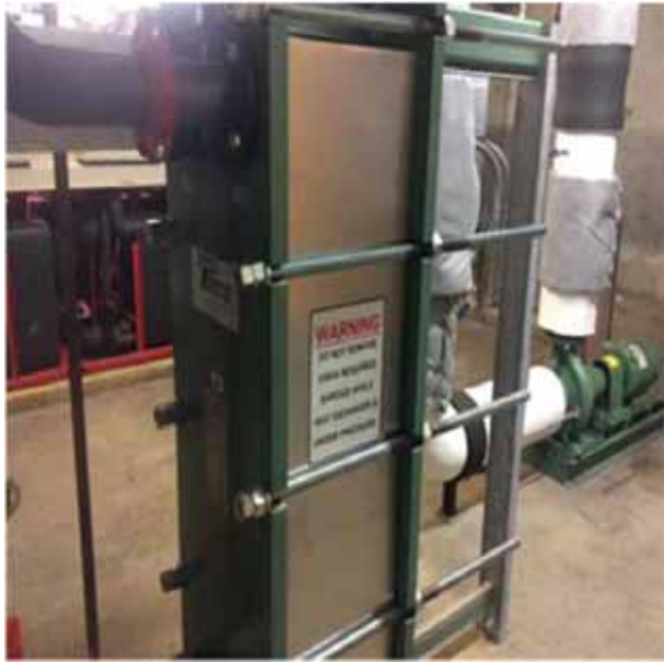
D3045 Chilled Water Distribution.2:- View of the heat exchanger unit.
