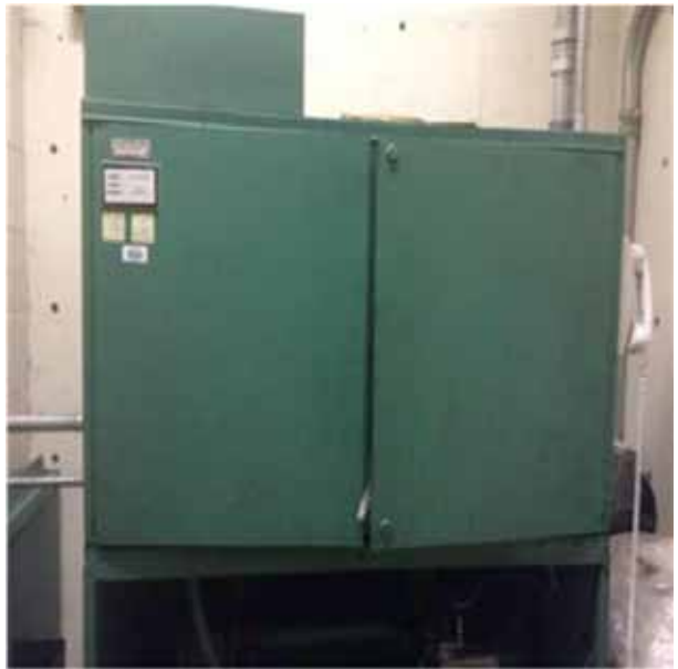
D1011 Passenger Elevators.3:- View of the hydraulic elevator equipment.
