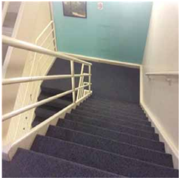
C2011 Regular Stairs.1:- View of typical steel stairs with carpet finish and metal handrails.
