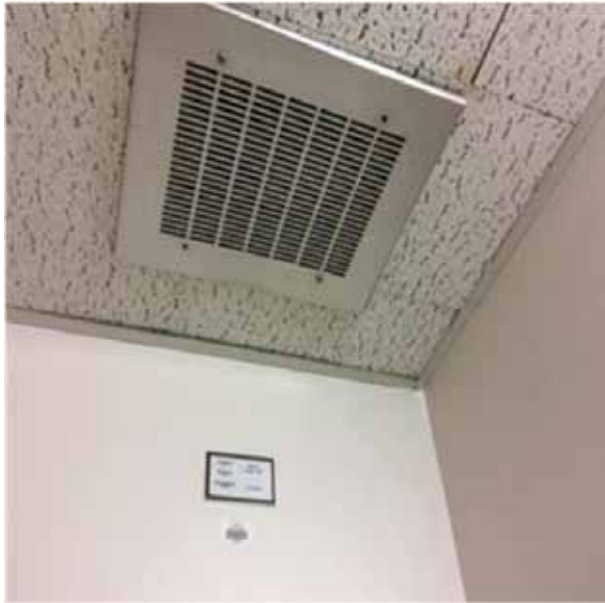
D3042 Exhaust Ventilation Systems.2:- View of a small capacity restroom exhaust fan unit.
