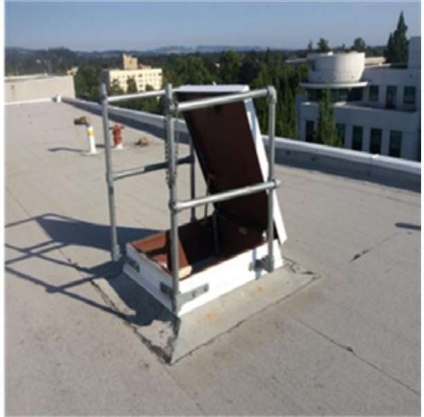
B3022 Roof Hatches.1:- View of typical galvanized roof hatch.
