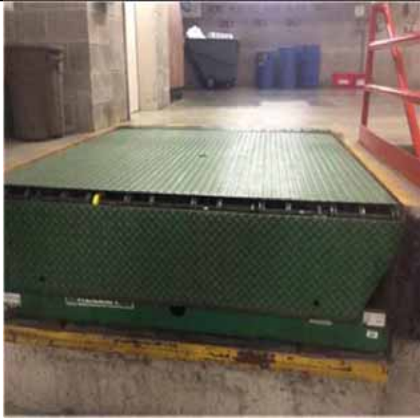
D1013 Lifts.1:- View of one of the dock levelers.
