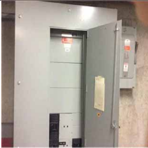
D5012 Low Tension Service & Dist.2:- View of secondary distribution panel EC2.
