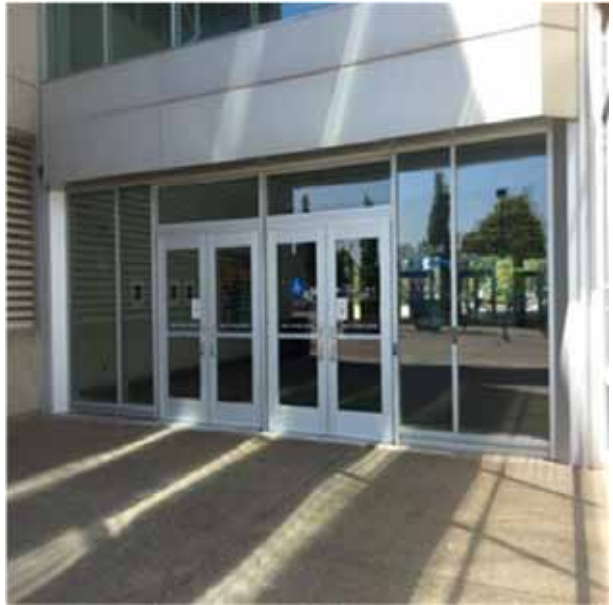
B2031 Glazed Doors & Entrances.2:- View of typical aluminum glazed doors.
