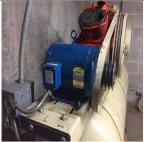
D2099 Other Piping Systems.2:- View of HVAC compressor 02.
