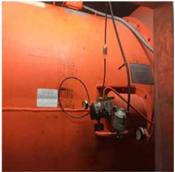
D3041 Air Distribution Systems.3:- View of return fan RF-07.
