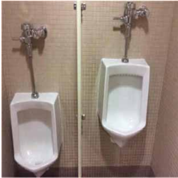
D2012 Urinals.1:- View of the wall mounted urinals.
