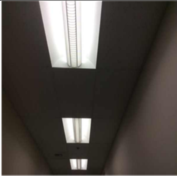
D5022 Lighting Equipment.1:- View of the 2' x 4' light fixtures.
