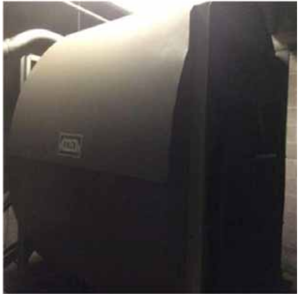
D3042 Exhaust Ventilation Systems.3:- View of one of the garage exhaust fan units.
