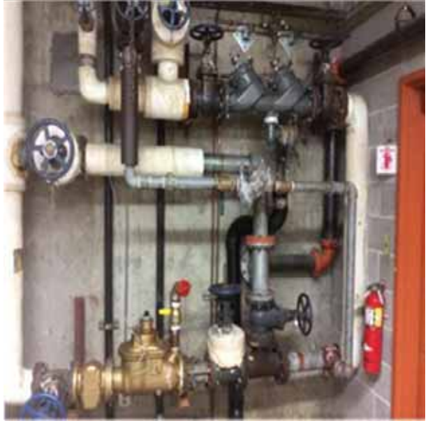
D2021 Cold Water Service.1:- View of the cold water supply system.
