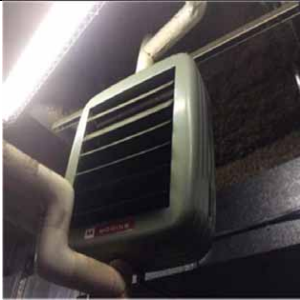
D3023 Auxiliary Equipment. 1:- View of the hot water unit heater.
