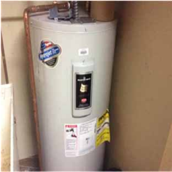
D2022 Hot Water Service.1:- View of domestic water heater DWH-01.
