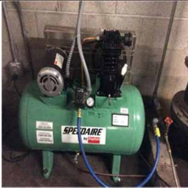
D2099 Other Piping Systems.1:- View of the fire compressor unit.
