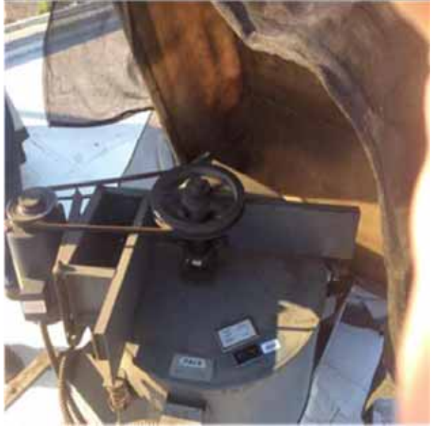
D3042 Exhaust Ventilation Systems.1:- View of one of the roof level exhaust fan units.
