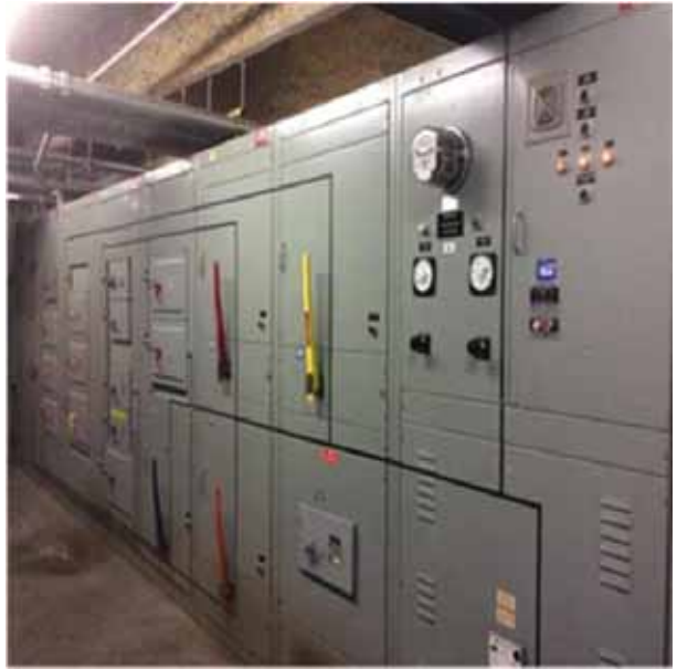
D5012 Low Tension Service & Dist.1:- View of the 480/277 voltage MDP.
