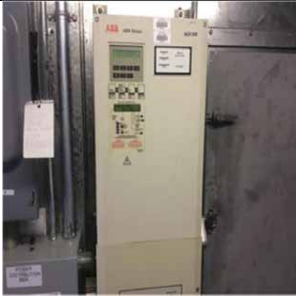
D3069 Other Controls & Instrumentation.1:- View of the ABB type VFDs.
