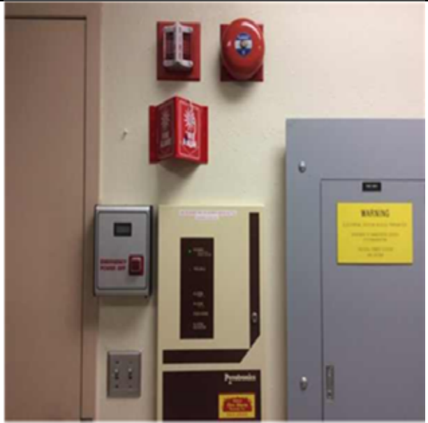
D4091 Carbon Dioxide Systems.2:- View of the control panel.
