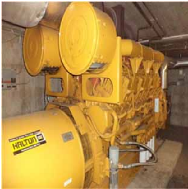
G4092 Site Emergency Power Generation.1:- View of the emergency generator.
