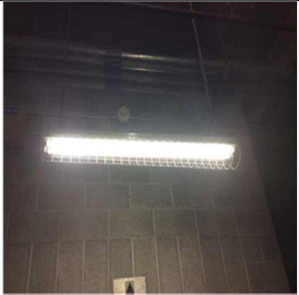
D5022 Lighting Equipment.2:- View of the strip light fixtures.
