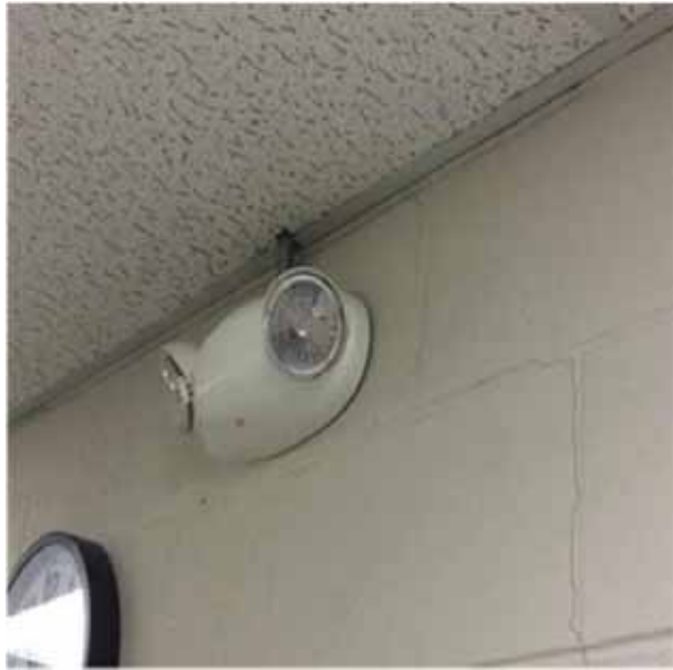
D5092 Emergency Light & Power Systems.1:- View of one of the emergency light fixtures.
