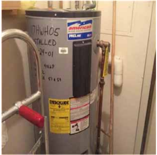
D2022 Hot Water Service.2:- View of domestic water heater DHW-05.
