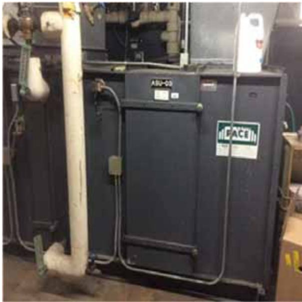
D3041 Air Distribution Systems.2:- View of AHU ASU-03.
