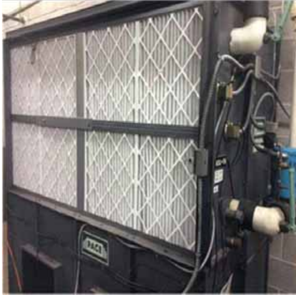
D3041 Air Distribution Systems.4:- View of water cooled fan coil unit ASU-11A and 11B.
