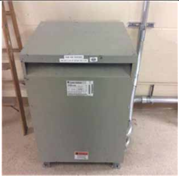
D5012 Low Tension Service & Dist.3:- View of a 75 KVA transformer.
