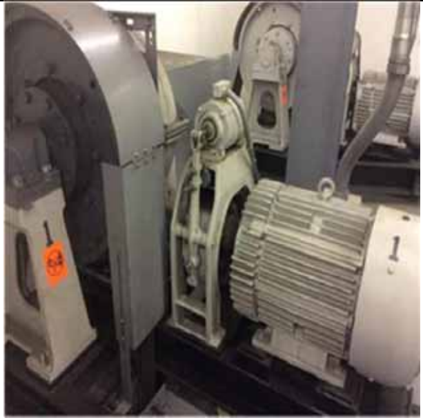
D1011 Passenger Elevators.1:- View of the hoist equipment at elevator 01P.
