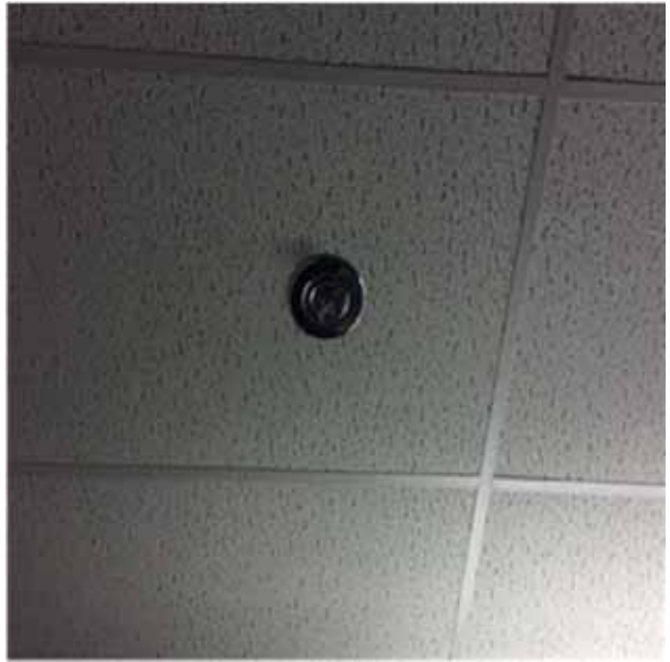
D4011 Sprinkler Water Supply.2:- View of a typical sprinkler head.
