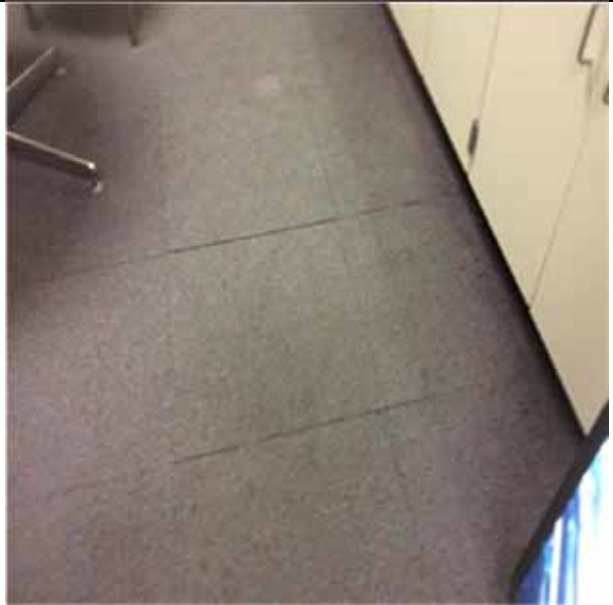
C3025 Carpeting.1:- View of typical carpet tiles.
