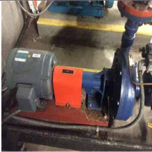
D3044 Hot Water Distribution.1:- View of pump/motor HWP-01.
