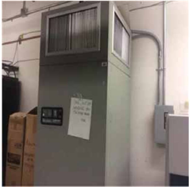
D3032 Direct Expansion Systems.1:- View of the indoor unit of the Liebert split-system.
