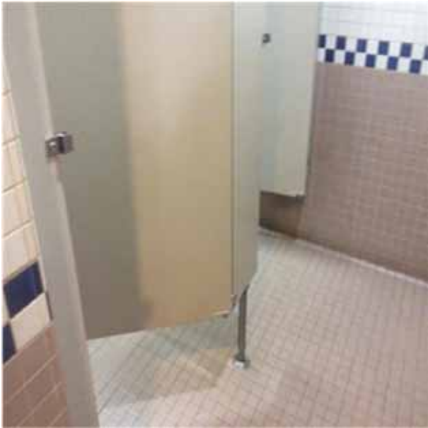
C1014 Site Built Toilet Partitions.1:- View of typical metal toilet partitions.
