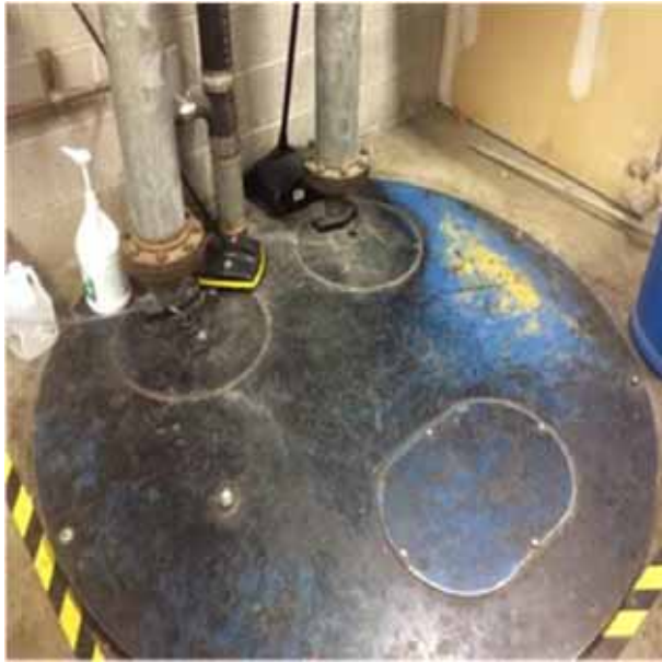
D2043 Rainwater Drainage Equipment.1:- View of one of the sump pump chambers.
