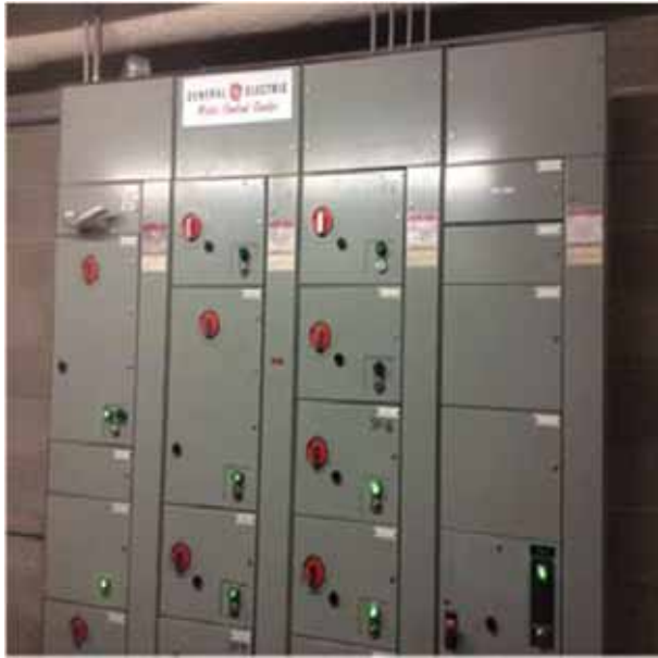
D5012 Low Tension Service & Dist.4:- View of MCC 1.
