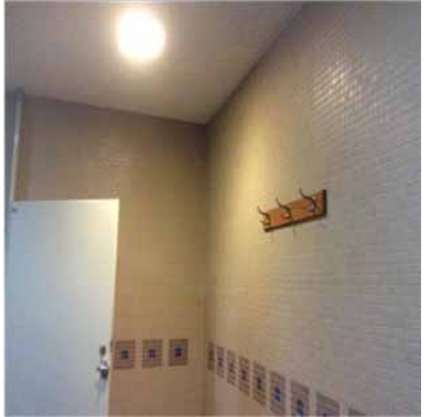
C3012 Wall Finishes to Interior Walls.2:- View of typical ceramic wall tiles.
