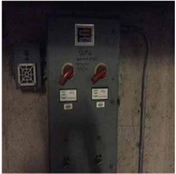
D2043 Rainwater Drainage Equipment.2:- View of one of the sump pump control panel units.
