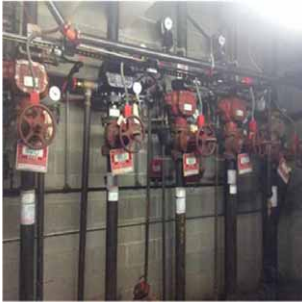
D4011 Sprinkler Water Supply.1:- View of the fire suppression system riser and valves.
