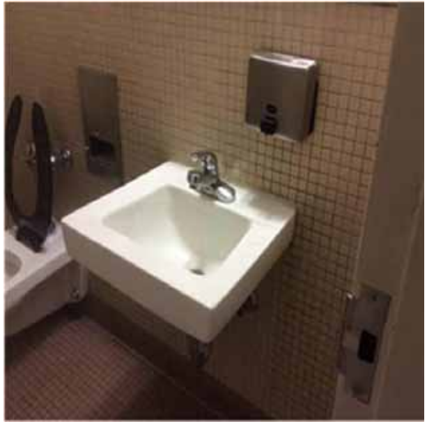
D2013 Lavatories.1:- View of one of the wall mounted lavatories.
