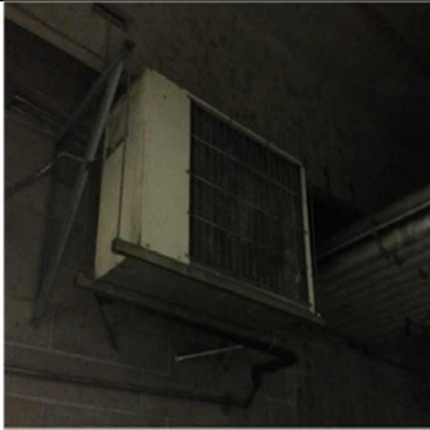
D3032 Direct Expansion Systems.2:- View of the outdoor unit of the Liebert split-system.
