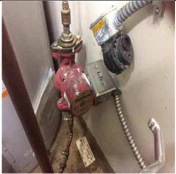
D2023 Domestic Water Supply Equipment.1:- View of a domestic water circulation pump/motor.
