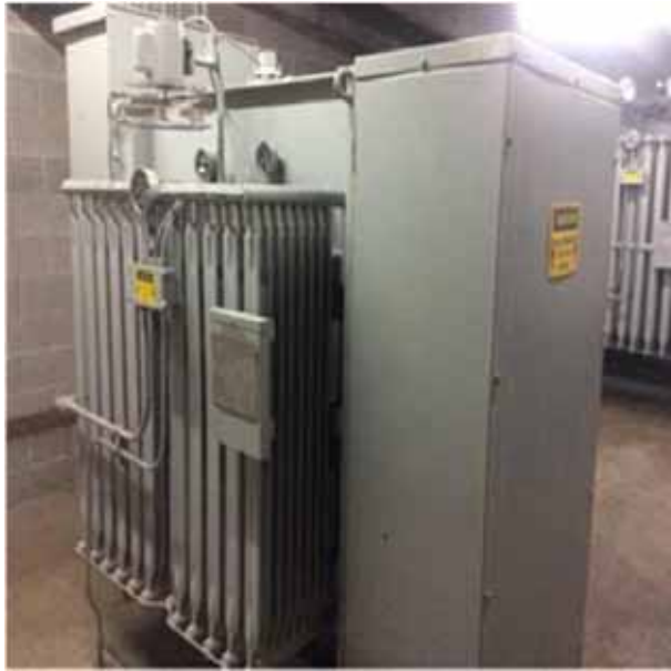
D5011 High Tension Service & Dist.1:- View of one of the main transformers.
