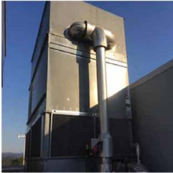
D3031 Chilled Water Systems.2:- View of cooling tower CT-01.
