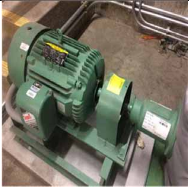
D3045 Chilled Water Distribution.1:- View of chilled water pump/motor CWP-01.
