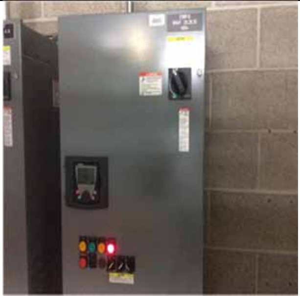
D3069 Other Controls & Instrumentation.2:- View of the newer GE type VFDs.
