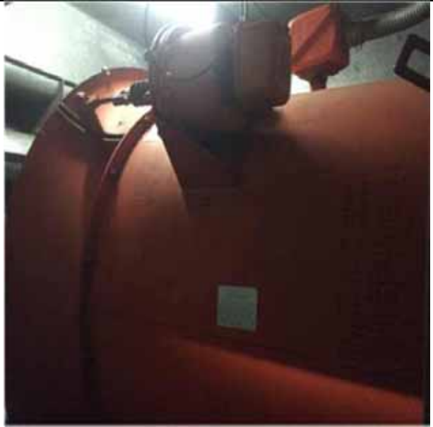
D3041 Air Distribution Systems.1:- View of supply fan SF-02.
