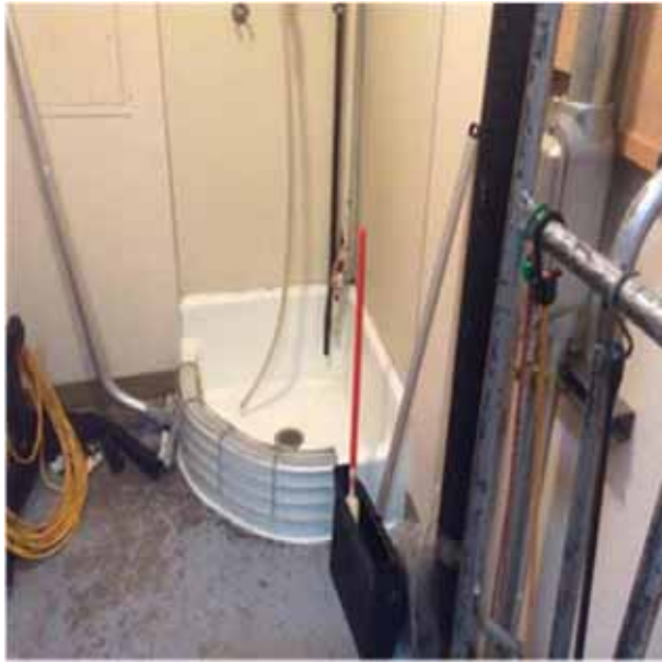
D2014 Sinks.2:- View of the custodial sink.
