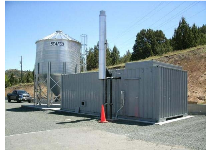
Biomass Boiler at Blue Mountain Hospital, John Day
