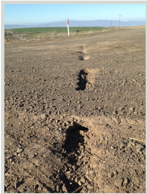
Example of a poorly repaired utility line on a Sherman County gravel road.
