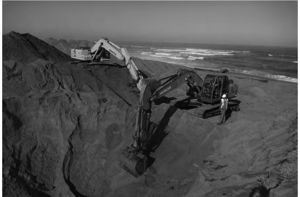
Biggest sand toys ever. Excavators were used to remove rhizomes and to bury sand contaminated with rhizomes deeply enough that it could not regenerate.
