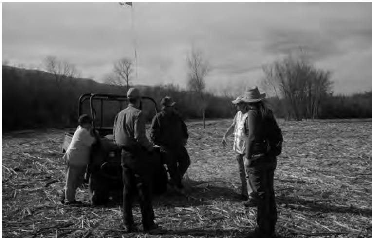
Dense Arundo donax stands in the Salinas River (above) and stream land management crew conferring next to the arundo mower with widespread mulched arundo canes (below). Photos by Paul Robins
