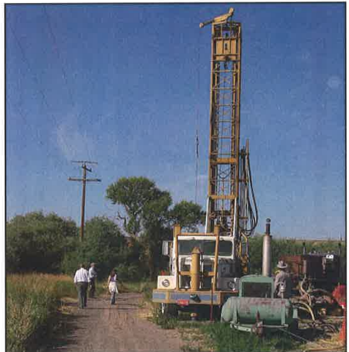
Klamath County drilled a new injection well for geothermal heated water that heated Henley High School. The project was paid in part with Recovery Act (stimulus) funds.
