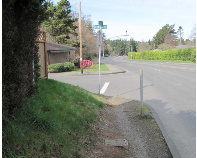
Missing sidewalk creates a barrier for pedestrians and is not accessible for all users.
