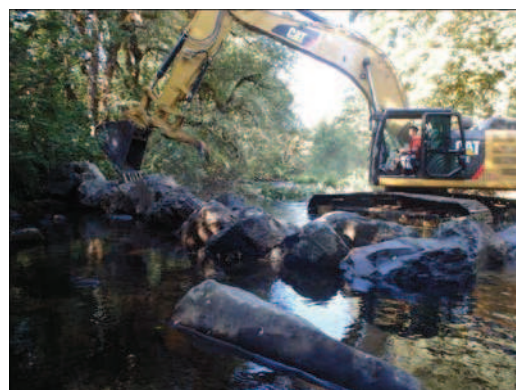
Contractor placing boulders on an in-stream habitat project on Little Fall Creek.
