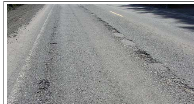
Pavement Condition: Poor
