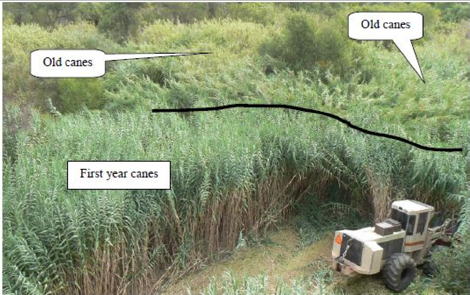
Figure 2-6. First year Arundo canes at full height (6+ m). The tractor is 10' high. This area had been cut as a fuel break the year before and is being cut again. Energy stored in rhizomes underground allow this rapid regrowth after cutting or fire events. Note simple unbranched vertical structure, very high cane density, and deep green color of the new, resprouted canes. Older canes in the background are less vertical and are a more yellowish color.
