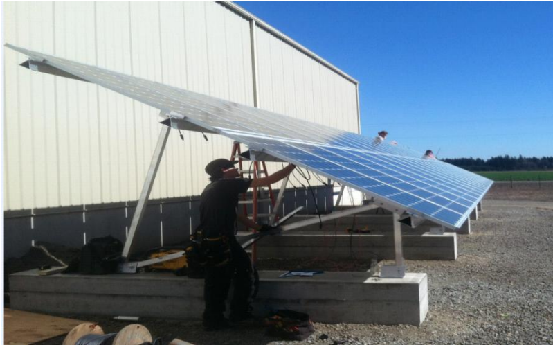
Installation of 10Kw array at Mullen Farms St. Paul, OR Made possible by Oregon Feed-In-Tariff Pilot Program
