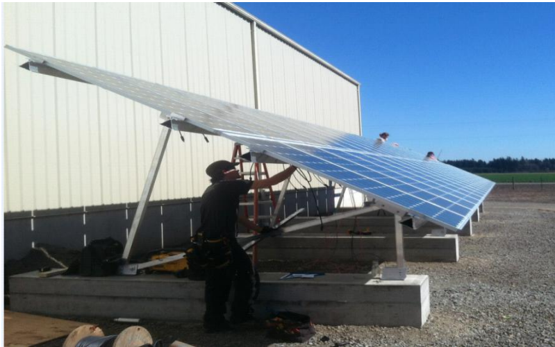
Installation of 10Kw array at Mullen Farms St. Paul, OR Made possible by Oregon Feed-In-Tariff Pilot Program
